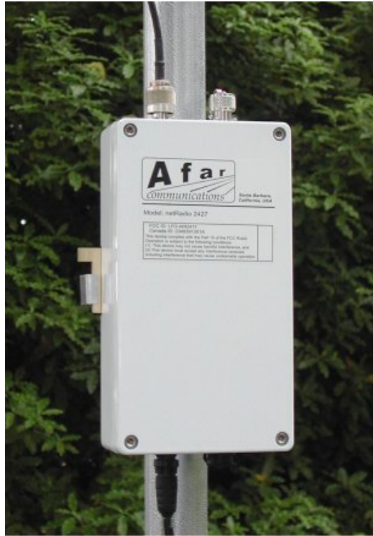
Figure 1.1: Pole Mounted Radio
